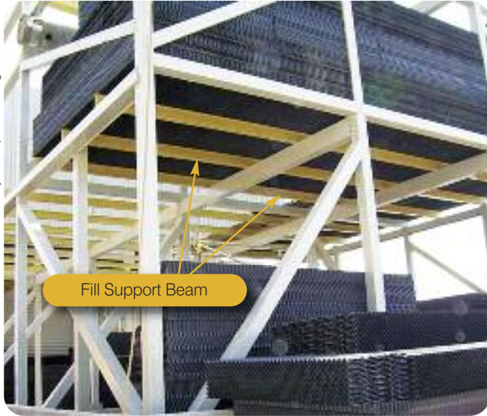
Composite cooling tower fill support beam
